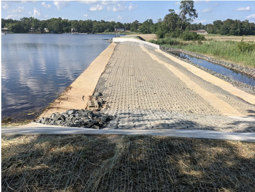
Figure 2. Secondary Spillway operating at normal pool level. Lake elevation 2" below upstream concrete apron
